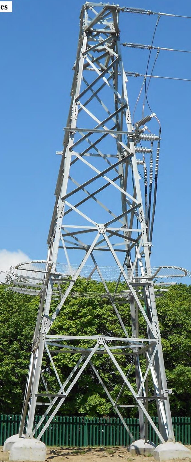
38kV Line Termination Mast Photograph Showing Typical 38kV Underground Cable to Overhead Line Terminations
