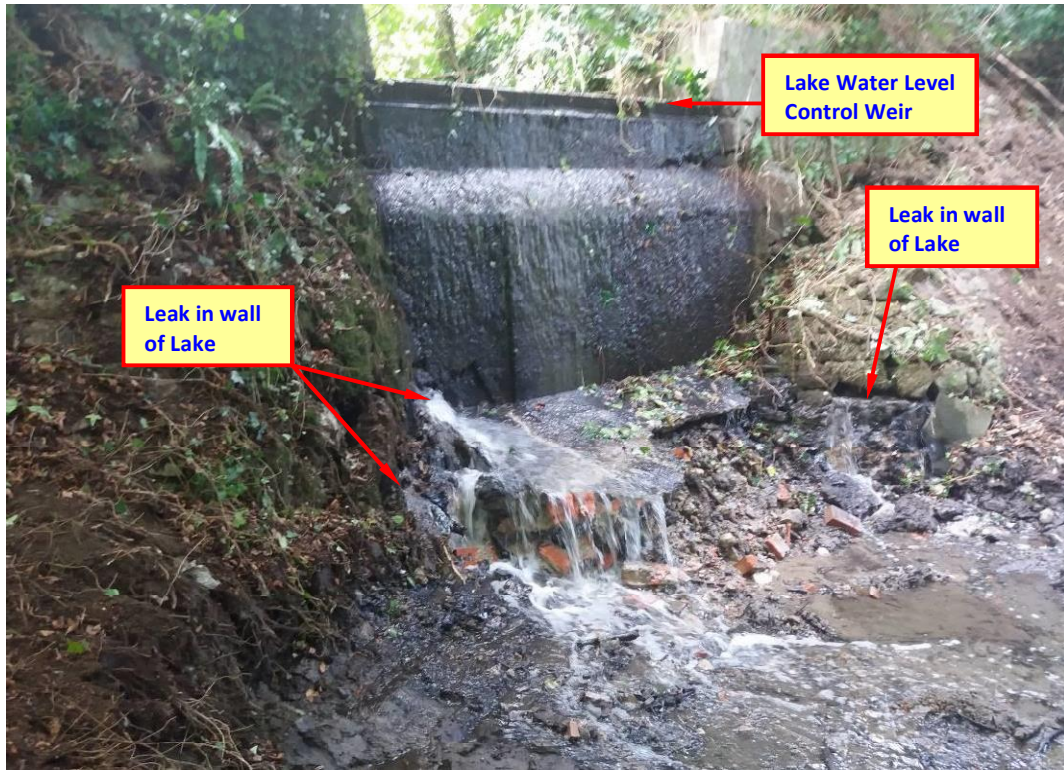
Figure 1 – Existing leak in lake wall at downstream end
